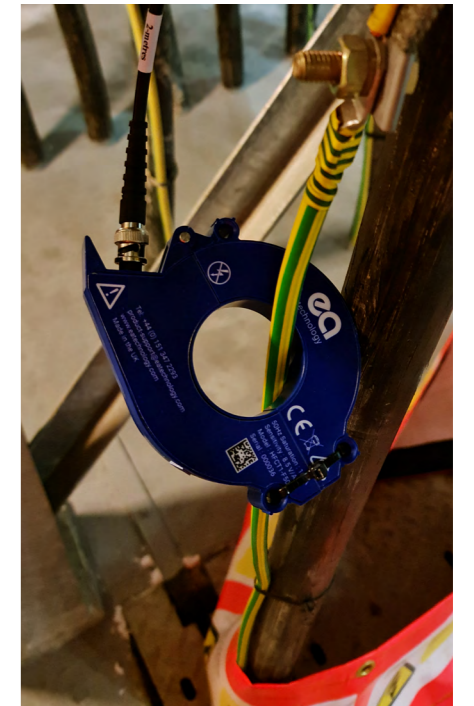
Figure 4: HFCT on earth braid of HV cable
