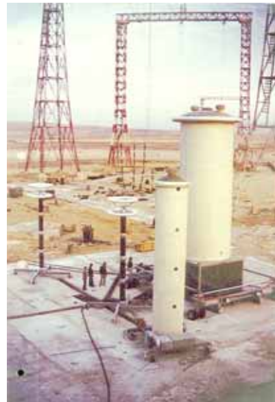
Outdoor impulse generator & multiple chopping gap 2400 kV
