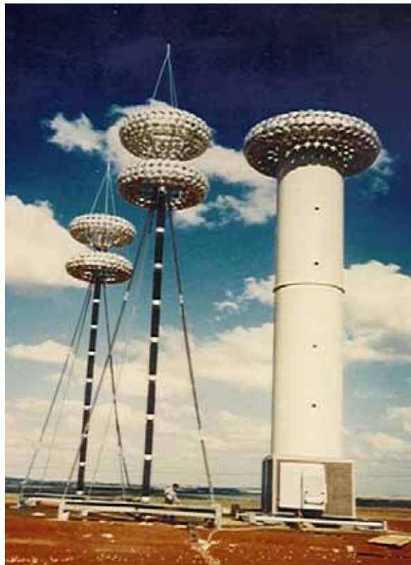
Outdoor test system X kV
