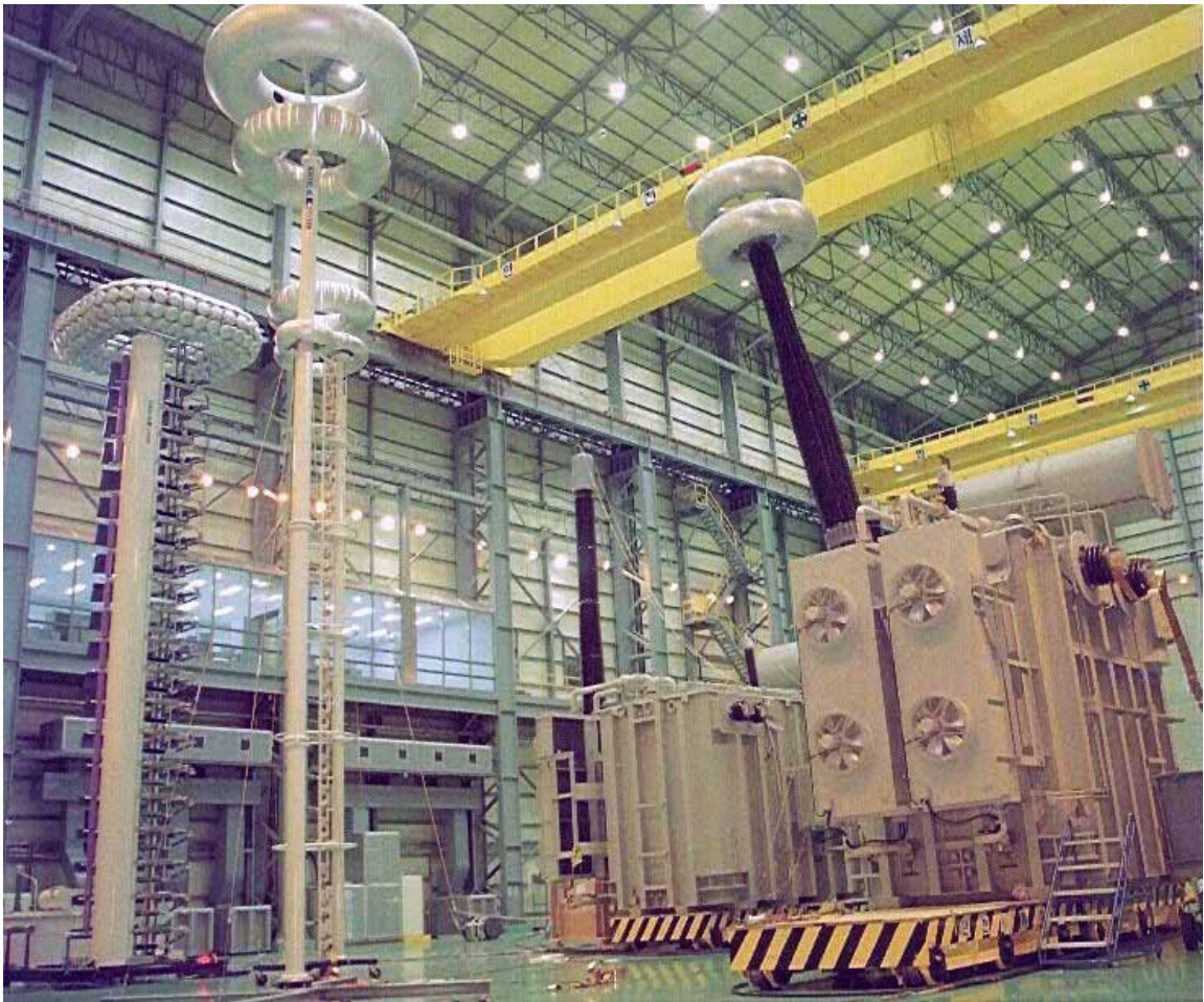
Impulse test system with 4000 kV impulse generator & divider and 3600 kV multiple chopping gap at Hyundai Heavy Industries, Ulsan, South Korea
