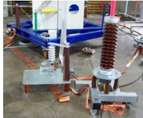
Impulse current testing arrangement for MV arresters
