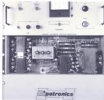
VIEW BEHIND ACCESS PANEL SHOWING VOLTAGE MONITOR RELAY AND CONTROL TRANSFORMERS
